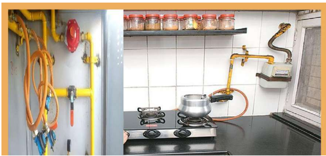
Photo No.11 CNG pipe line in the Kitchen
