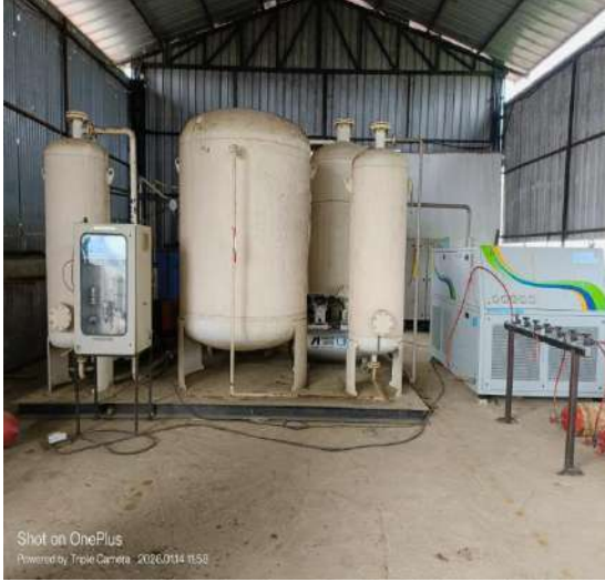
Photo No. 2 Biogas Purification & Compressor Unit
